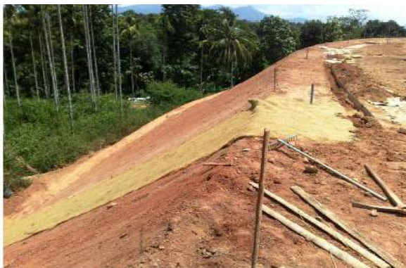
Fig. 4: a) Layering and fixing of coir ECB during vegetation of slopes and problem soil at Wayanad cricket
